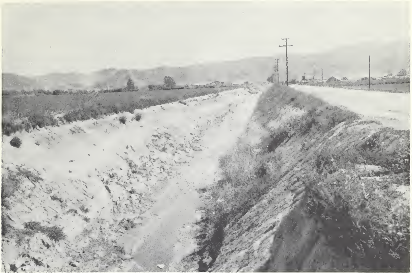
Photo 3. Miguelito Flood Channel, looking upstream from Central Avenue, showing sloughing along toes of channel excavation. Sloughing occurred in a layer of unstable silt clay material.
