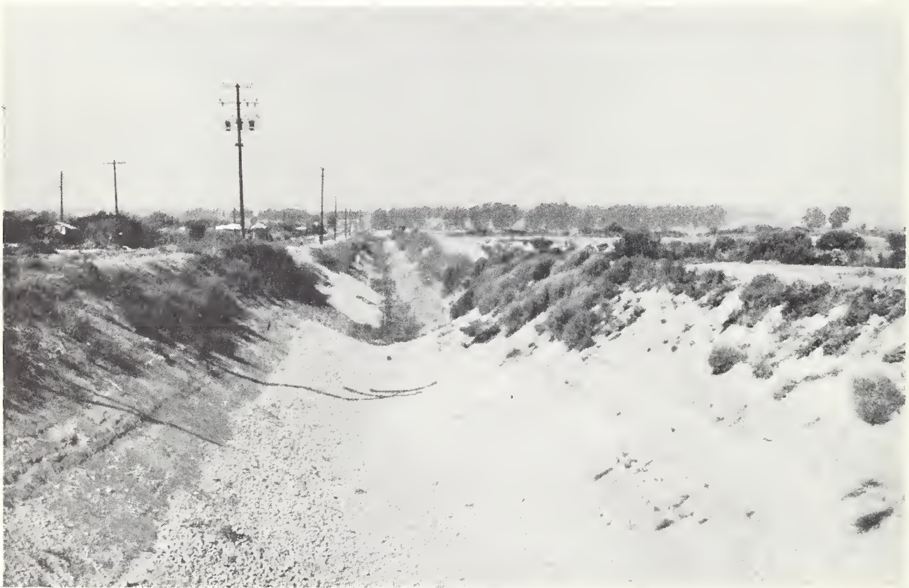
Photo 2. Miguelito Flood Channel, looking downstream from private vehicular bridge 1 mile south of Central Avenue, showing catenary shape of coarse loose rock fill in bottom of the channel.
