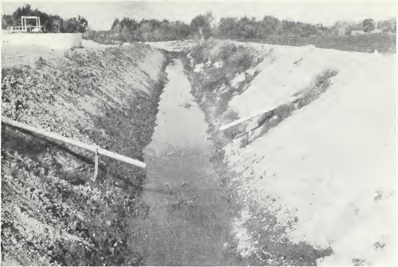
Photo 8. Miguelito Flood Channel, view looking downstream from Central Avenue, showing unstable nature of channel bottom material.
