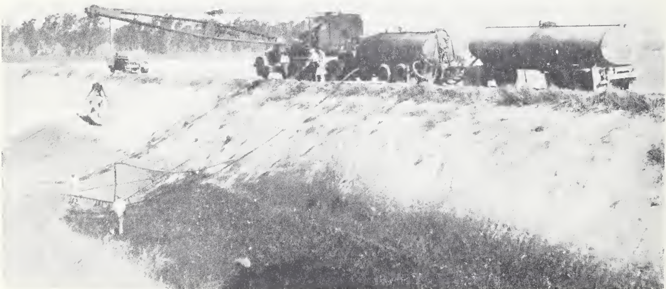
Photo 7. Miguelito Flood Channel, view showing use of clam bucket to move asphalt spray bar.
