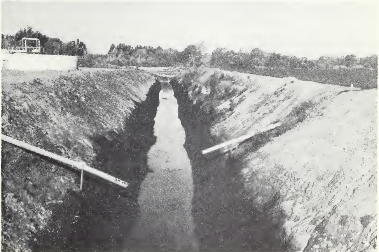
Photo 9. Miguelito Flood Channel, looking downstream from Central Avenue, showing condition of channel immediately after application of coarse gravel and application of emulsified asphalt binding material.
