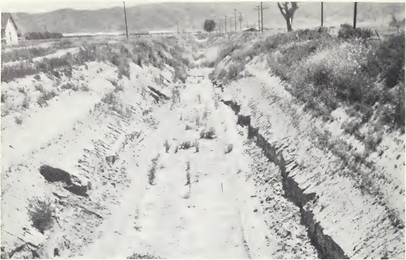
Photo 1. Miguelito Flood Channel, looking upstream from private vehicular bridge 1 mile south of Central Avenue, showing erosion damage to toe of earth section. This damage developed in a thick layer of non-cohesive material near channel grade.
