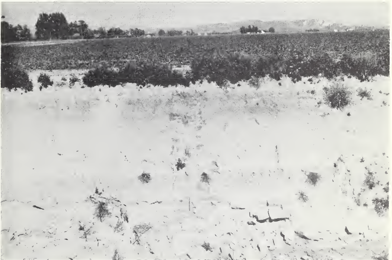
Photo 4. Miguelito Flood Channel, view taken immediately above Central Avenue, showing nature of fracture in silt clay layer. See Photo 3 above.
