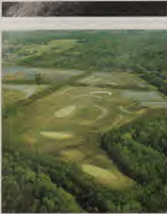
Mechanical excavation increases microtopographic complexity that benefits a diversity of wetland wildlife on WRP sites in the Arkansas River valley. (Kiah Gardner, Arkansas Game and Fish Commission)
