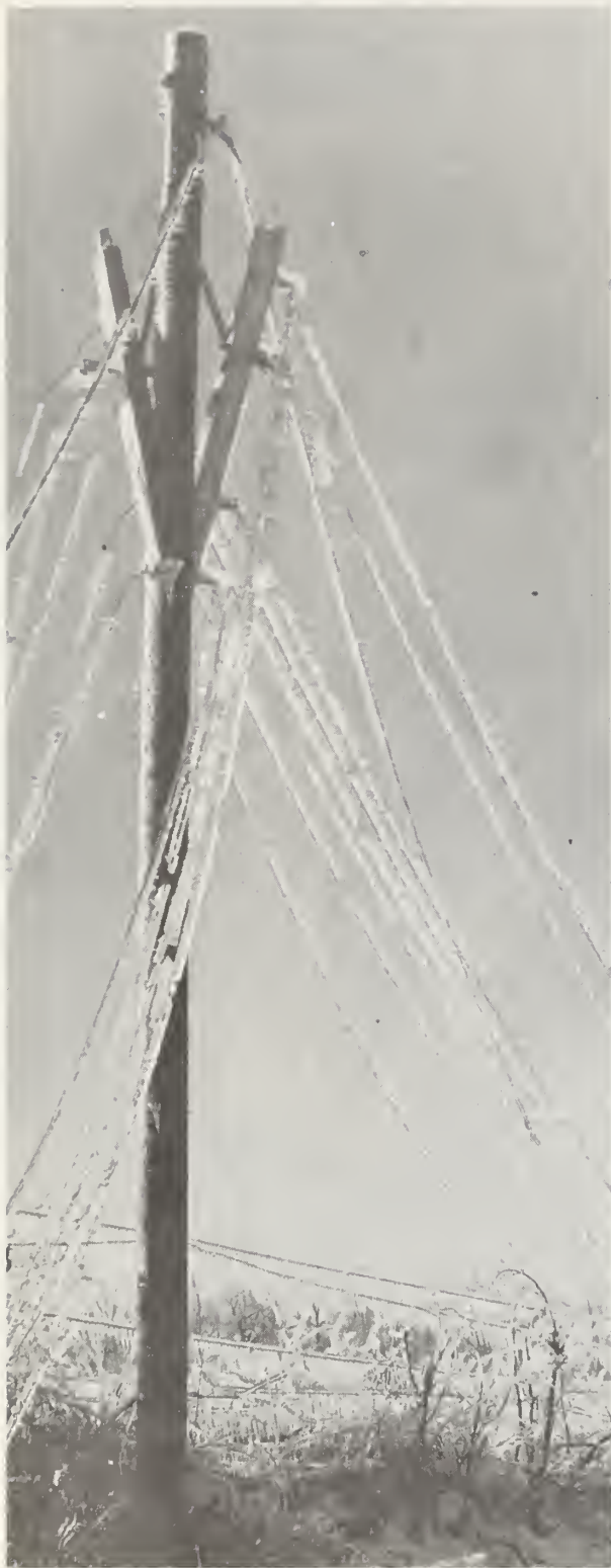
Burying telephone cables cuts construction costs, eliminates costly damage to lines from ice and wind storms.
