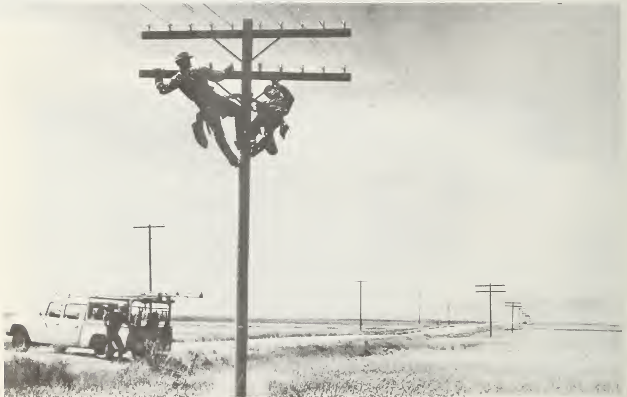
Poles followed country roads in many instances, to bring service to the "widest practicable number of rural users."
