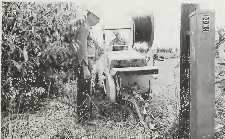
A narrow trench holds the wire pairs necessary to connect each subscriber to the larger cables.
