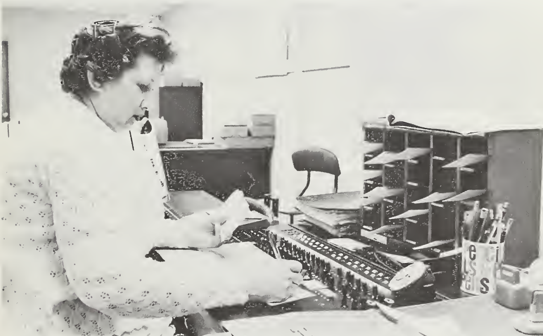
Switchboards are used by some rural telephone systems to provide directory assistance and toll service.
