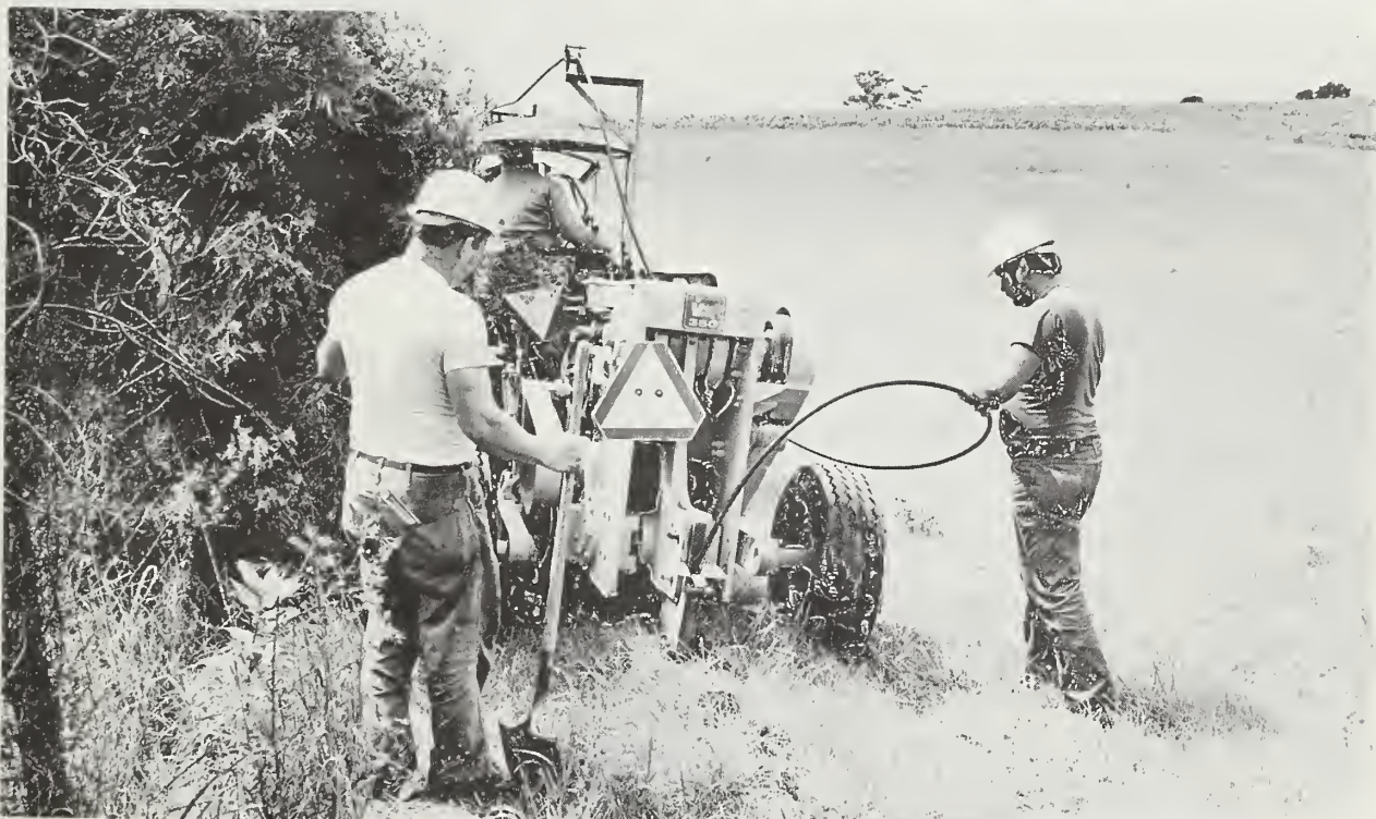
Fed through the blade of the plow, the cable is laid in a trench so narrow that little evidence shows after the plowing operation has been completed.
