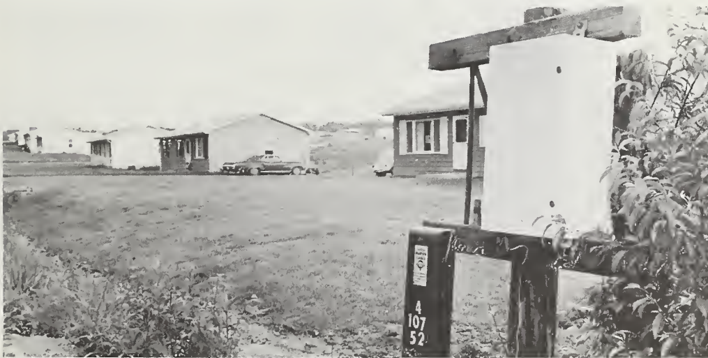
A telephone pedestal (numbers inscribed) permits connection of subscribers to underground telephone cables. The white cabinet contains subscriber carrier equipment which enables each pair of wires in the cable to be used for up to eight subscribers.
