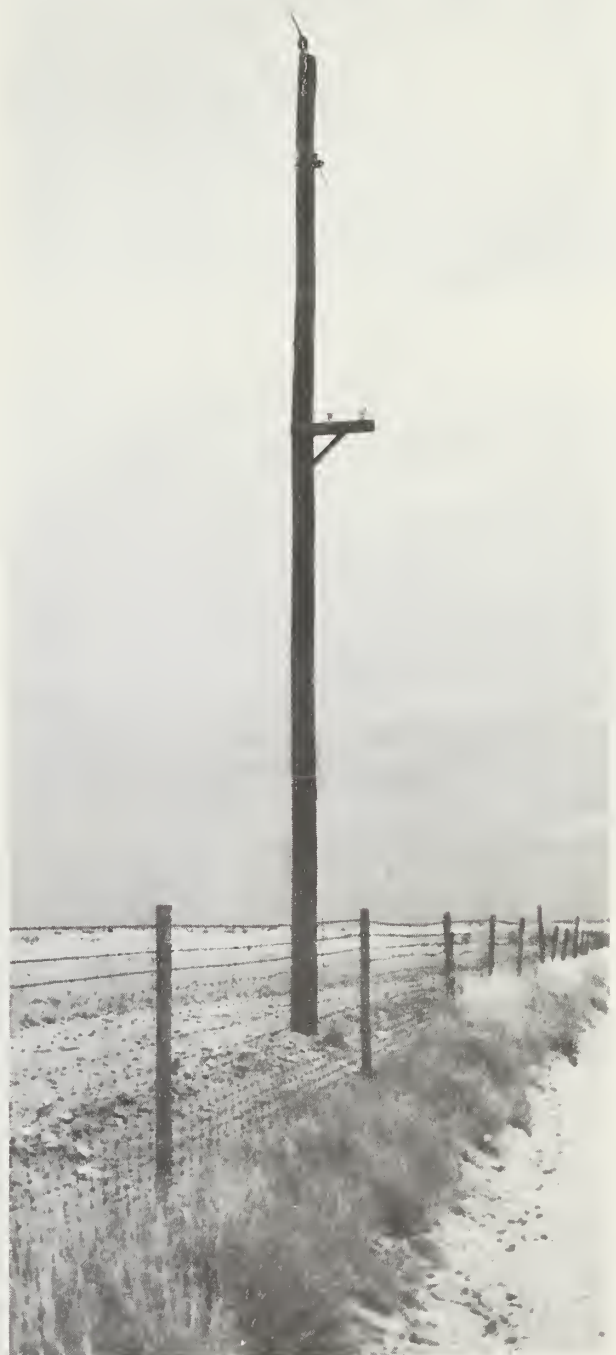
Joint-use of poles with electric suppliers was encouraged by REA as a cost-cutter. Many electric systems went farther and helped establish telephone systems.
