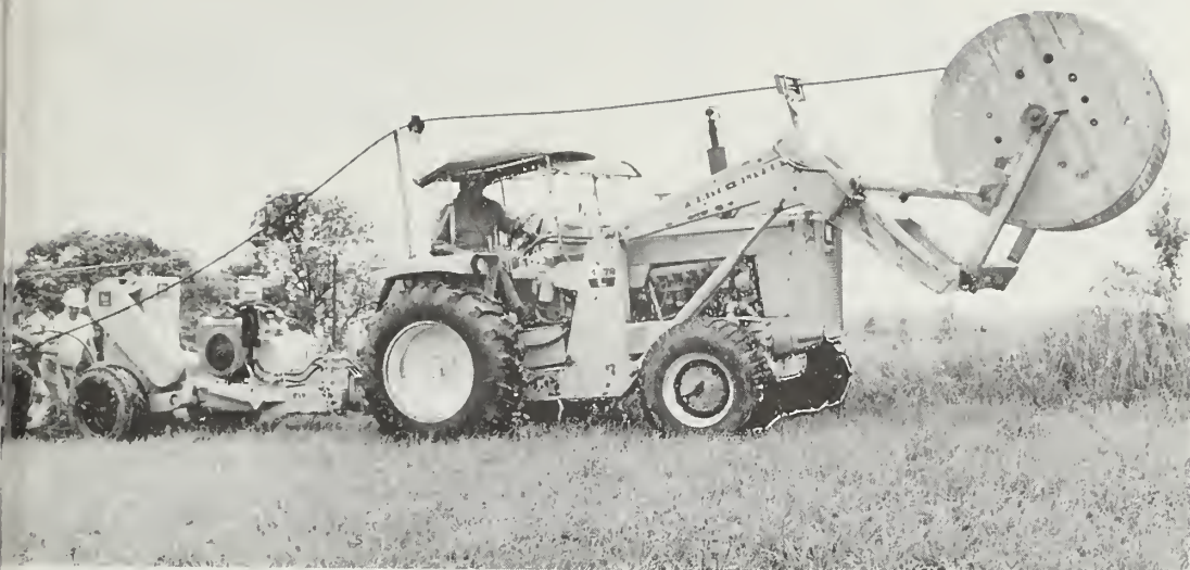
In one operation, specially designed equipment plows, buries and covers underground telephone cables.
