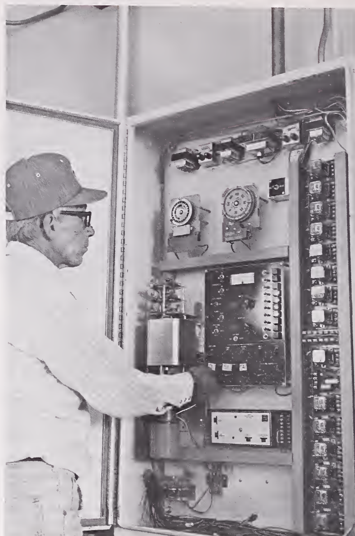
Figure 6-33. —Integrated heating and cooling control system with thermistor sensor. (Photo courtesy of Kansas Cooperative Extension Service.)
