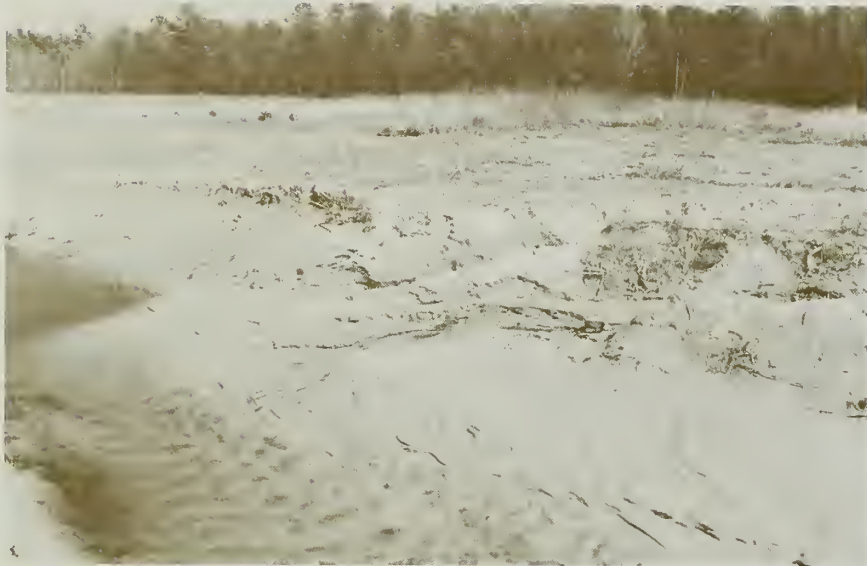
Improperly graded or seeded roadside ditch results in a severe erosion and sediment problem.
