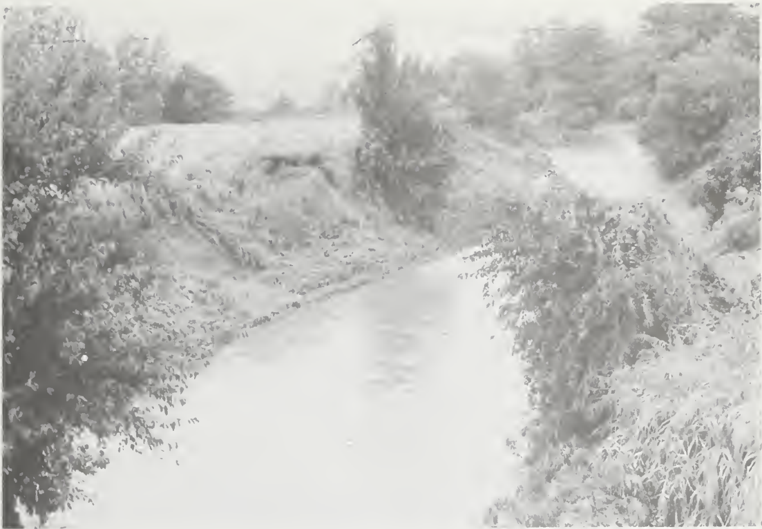
Photo 7 - Sloughing on channel banks
