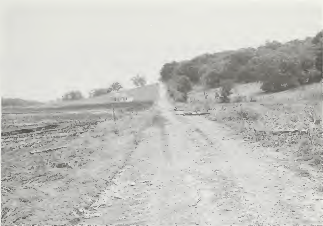
Photo 1 - Gravel washed off road and debris left on the road
