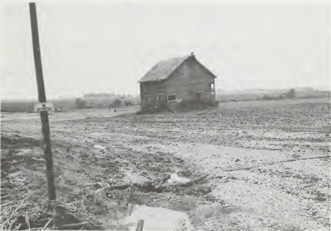
Photo 2 - Gravel from road and flood plain scour
