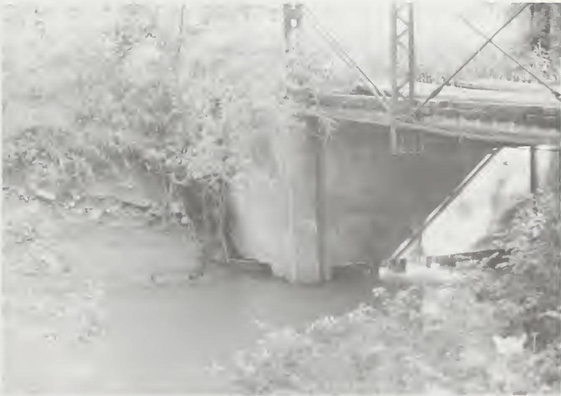
Photo 8 - Severe channel erosion has undercut concrete bridge abutment
