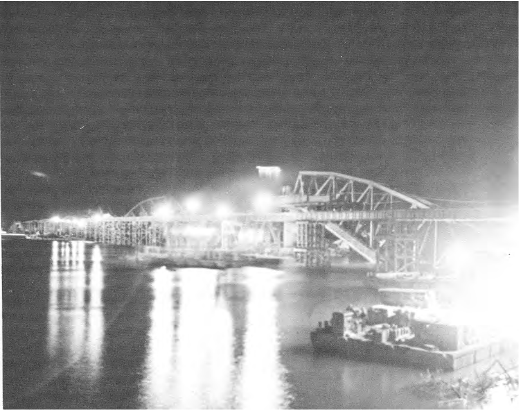
FRANKLIN D. ROOSEVELT MEMORIAL BRIDGE AT MAINZ. Construction proceeded day and night.
