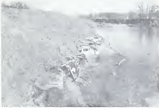
Figure 4.--Automobile bodies used to prevent undercutting of an embankment on the Washita River.
