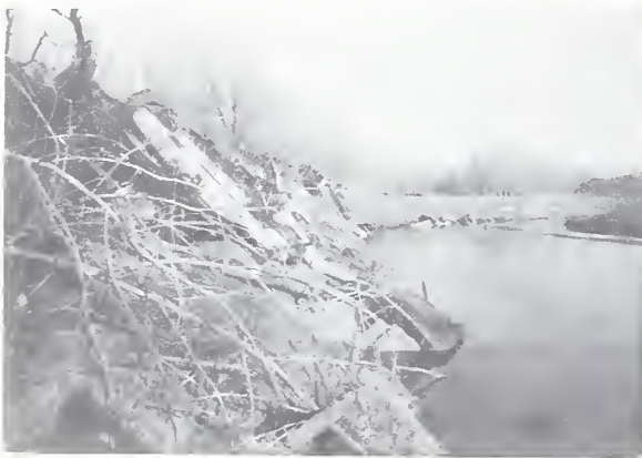
Figure 1.--Bank protection failure due to inadequate anchorage.
