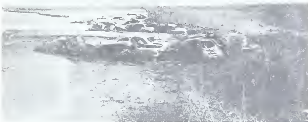
Figure 5.--Low-flow jetties constructed of well-anchored automobile bodies on the South Canadian River.
