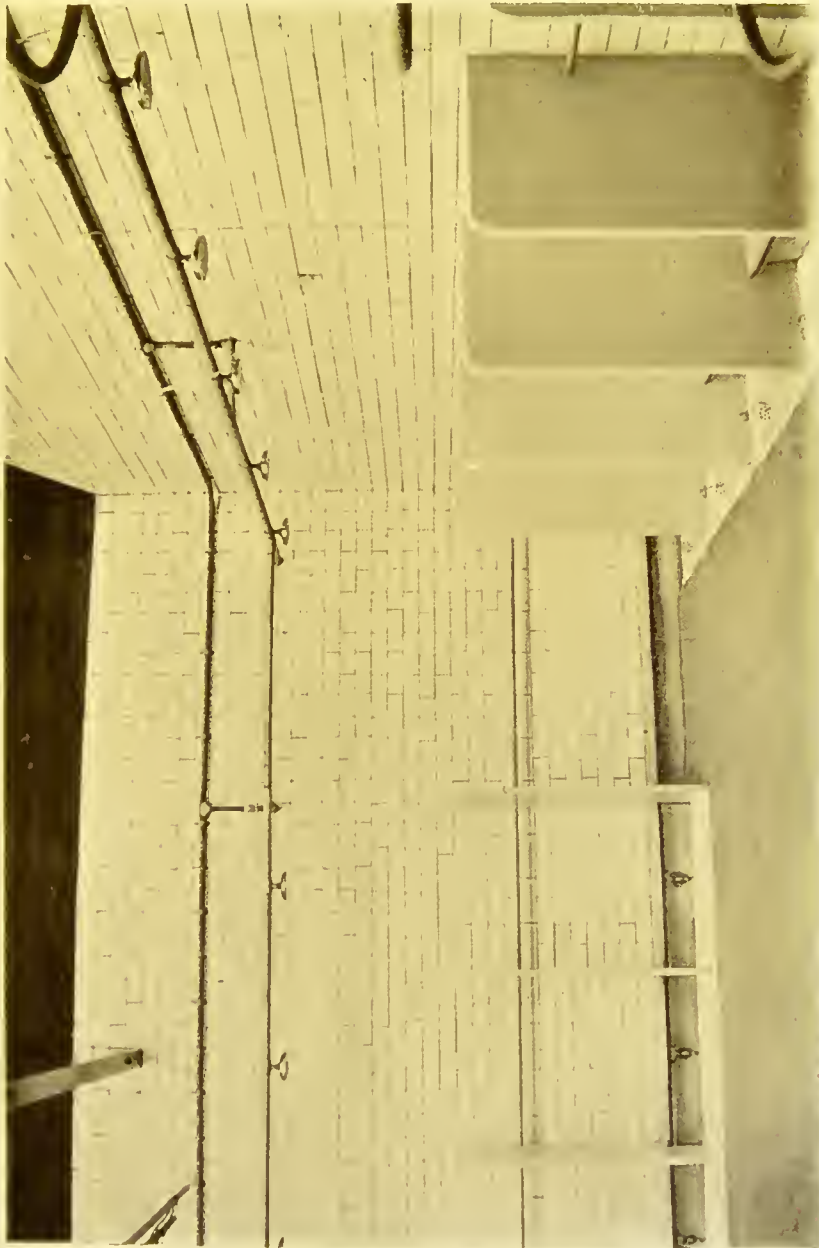
FIG. 9. SHOWER BATH INSTALLATION AT KNOLLS GREEN COUNTRY SCHOOL. (MANCHESTER EDUCATION AUTHORITY)
