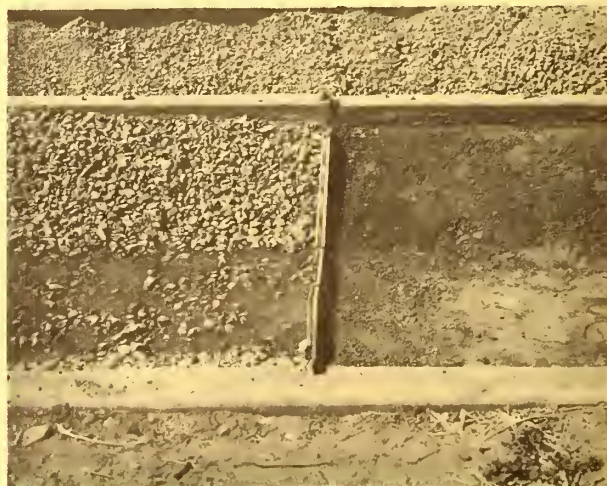
FIGURE 7. — An earth lining before covering with gravel is shown on the right. The lining to the left of the divider has been covered with gravel.
