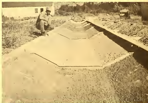
FIGURE 6. — Appearance of linings in channel C before covering with gravel. The lining in the foreground is C-8.
