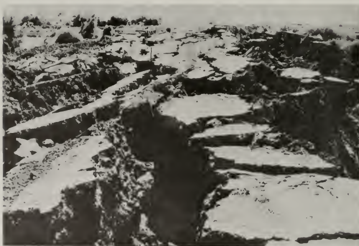
Levee Failure Caused by Foundation Shaking Imperial Valley Earthquake, May 18, 1940
