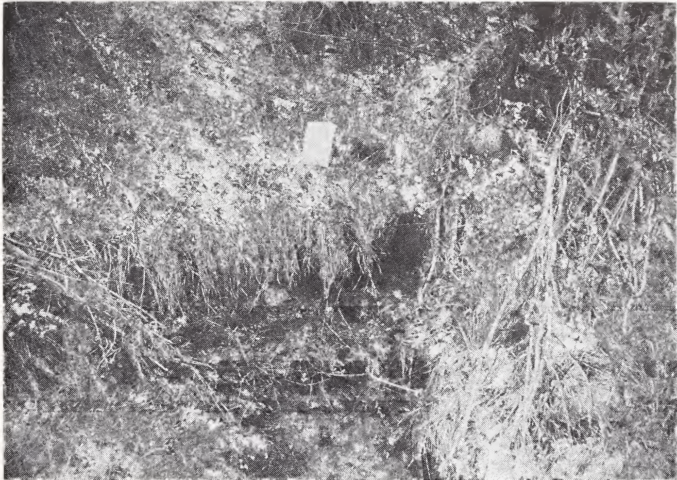
(PHOTO 5) Seepage at Right Abutment Toe.
