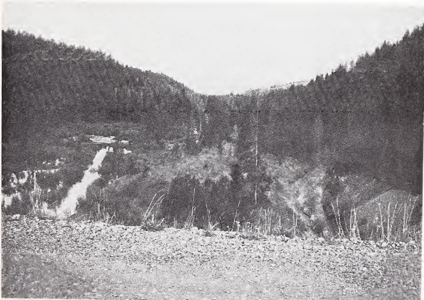
(PHOTO 6) Ponding Downstream of Embankment.
