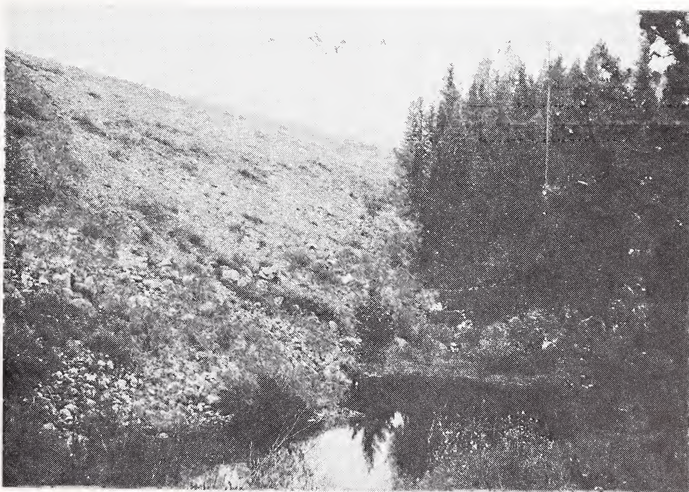
(PHOTO 4) Seepage at Downstream Slope near Left Abutment.
