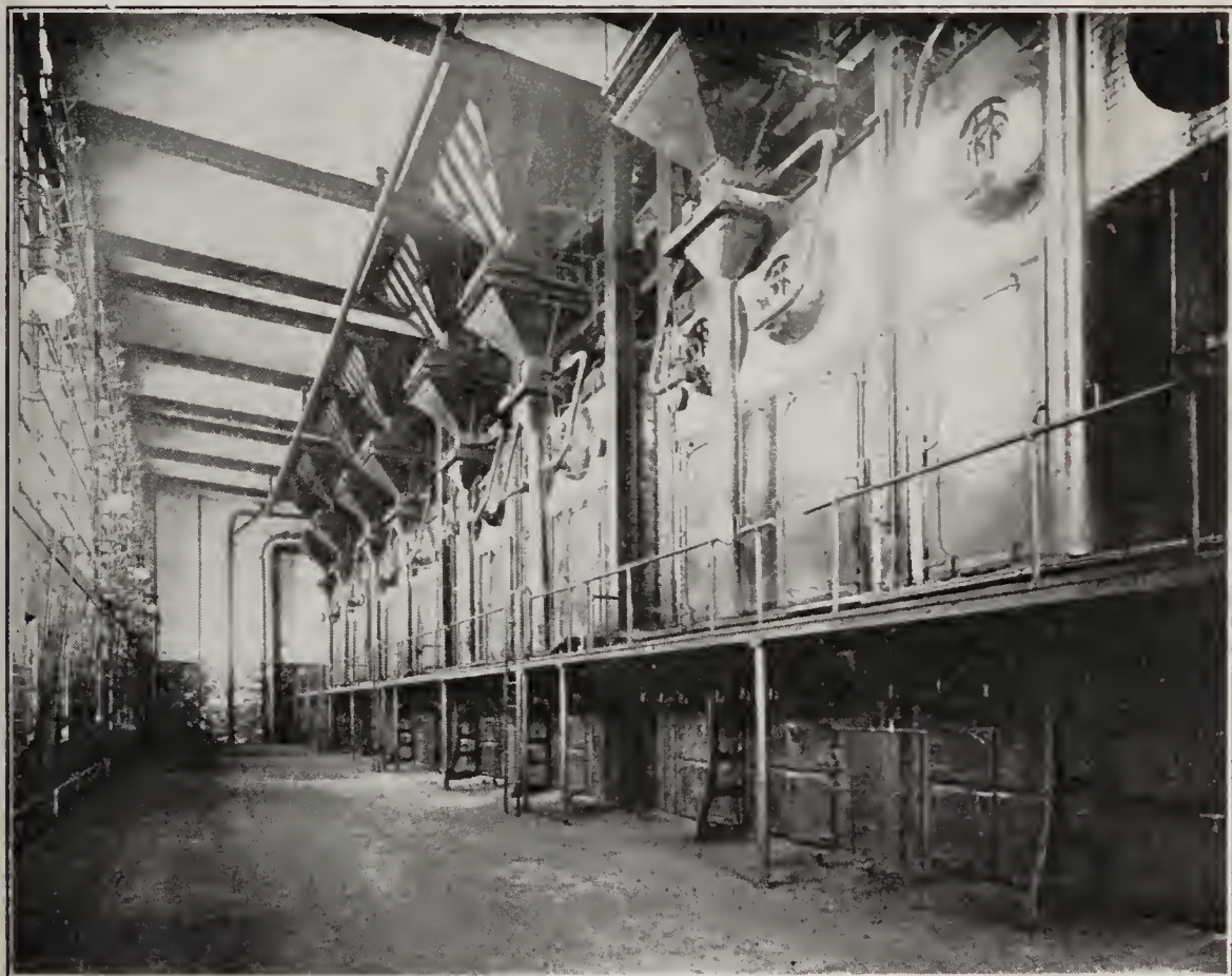
FIG. 288. — A battery of Babcock and Wilcox water-tube boilers. Coal bins above.
