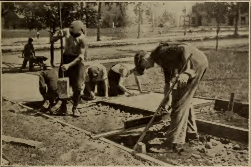
Illus. 11. Leveling Up Forms, Tamping the Undercoat, and Using the Jointer and Edger.
