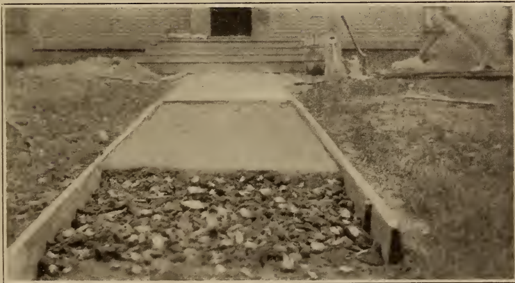
Illus. 10. Showing Gravel Sub-Base, Rough Concrete Undercoat and the Top or Finished Coat.
