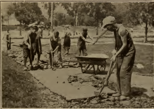
Illus. 9. Tearing Up Old Tar and Gravel Walk, Old Walk to Be Used as Large Aggregate in New Concrete Walk.
