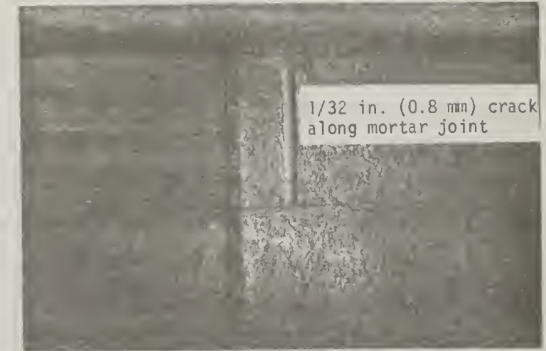
Fig. 3.3 Crack in a Hollow Block Wall Caused by Adjacent Excavation
