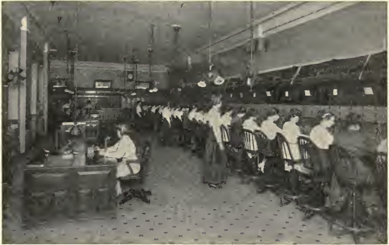
FIG 32.—Telephone central exchange
