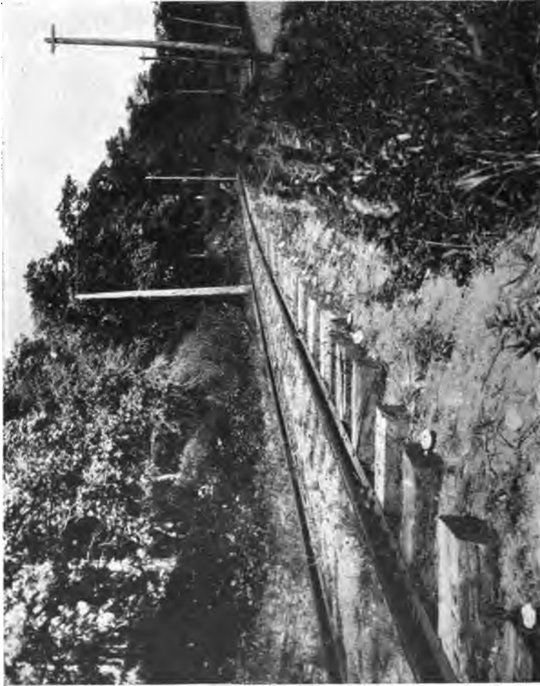
FIG. 116.—Fruiting bodies of a gill fungus (probably Lentinus lepideus ), on street railway ties. The mycelium of each of these is, of course, destroying the wood of the ties. Illustrates how prevalent the fungus may become on timbers placed under such conditions as those of ties. Photograph by Dr. F. Ramaley.
