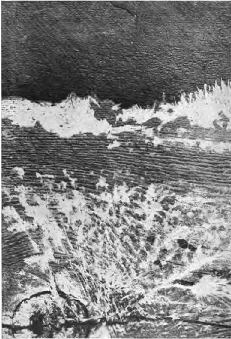
FIG. 121.—The dry-rot fungus ( Merulius lacrymans ). Shows the surface of a pine board which has been attacked by the dry-rot mycelium; it is not yet, however, completely converted to punk. The felted mycelium has been partially removed, showing the accentuated grain of the attacked portions. The mycelium has penetrated some distance beyond the white mycelial felt. Original.
