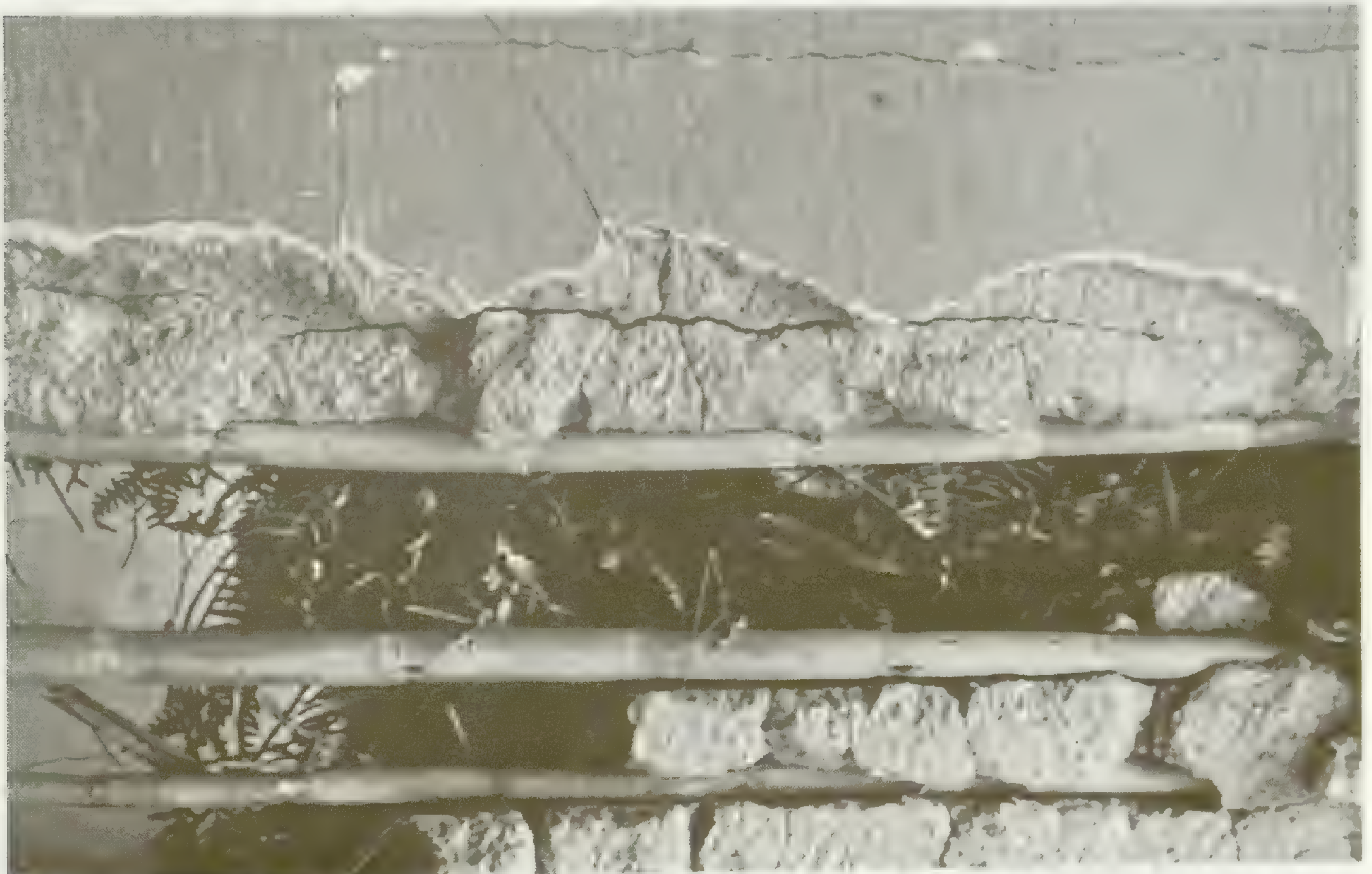
Internal structure of the disintegrating wall
