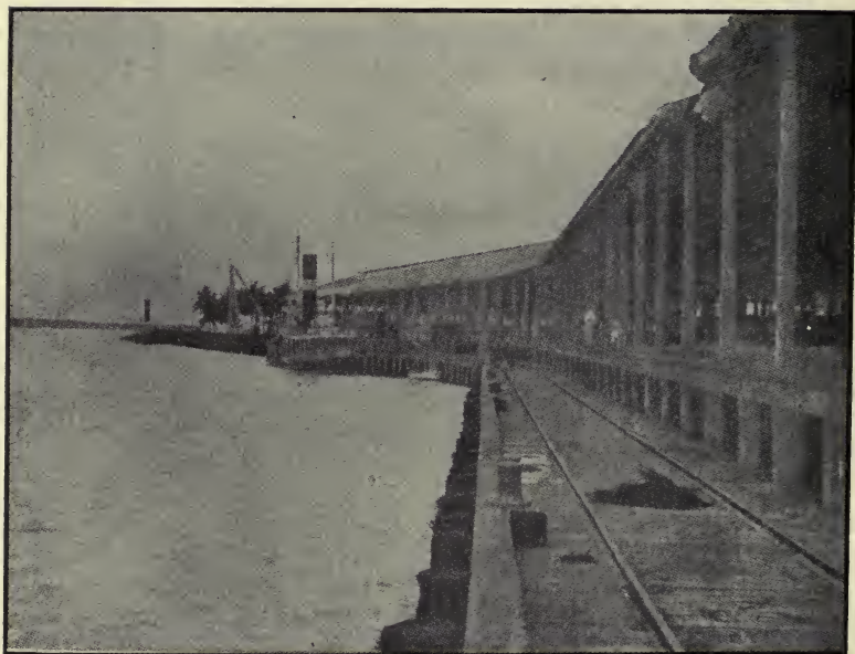
The New Wooden Pier at La Boca, on the Pacific, 800 feet long.
